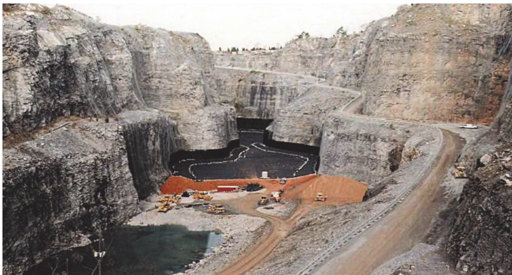
Figure 10 Landfill liner installation as part of landfill construction in a former quarry, Bristol, United Kingdom (Breitenbach, 2008)
